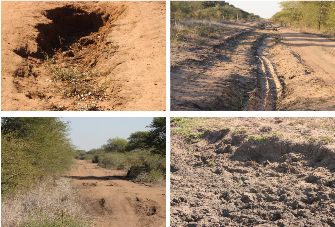
Figure 4 – Evident erosion signs along the pipeline
