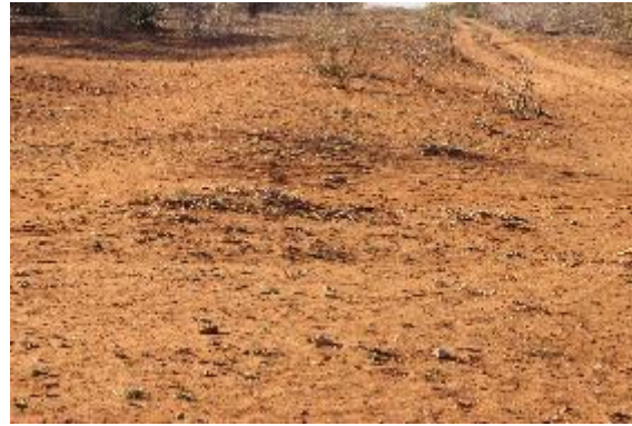
Figure 8 –Bare patches along the pipeline
